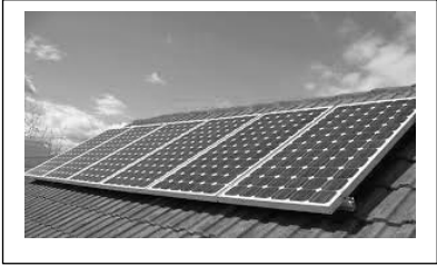
(ii) Solar power plant Stesen janakuasa solar
